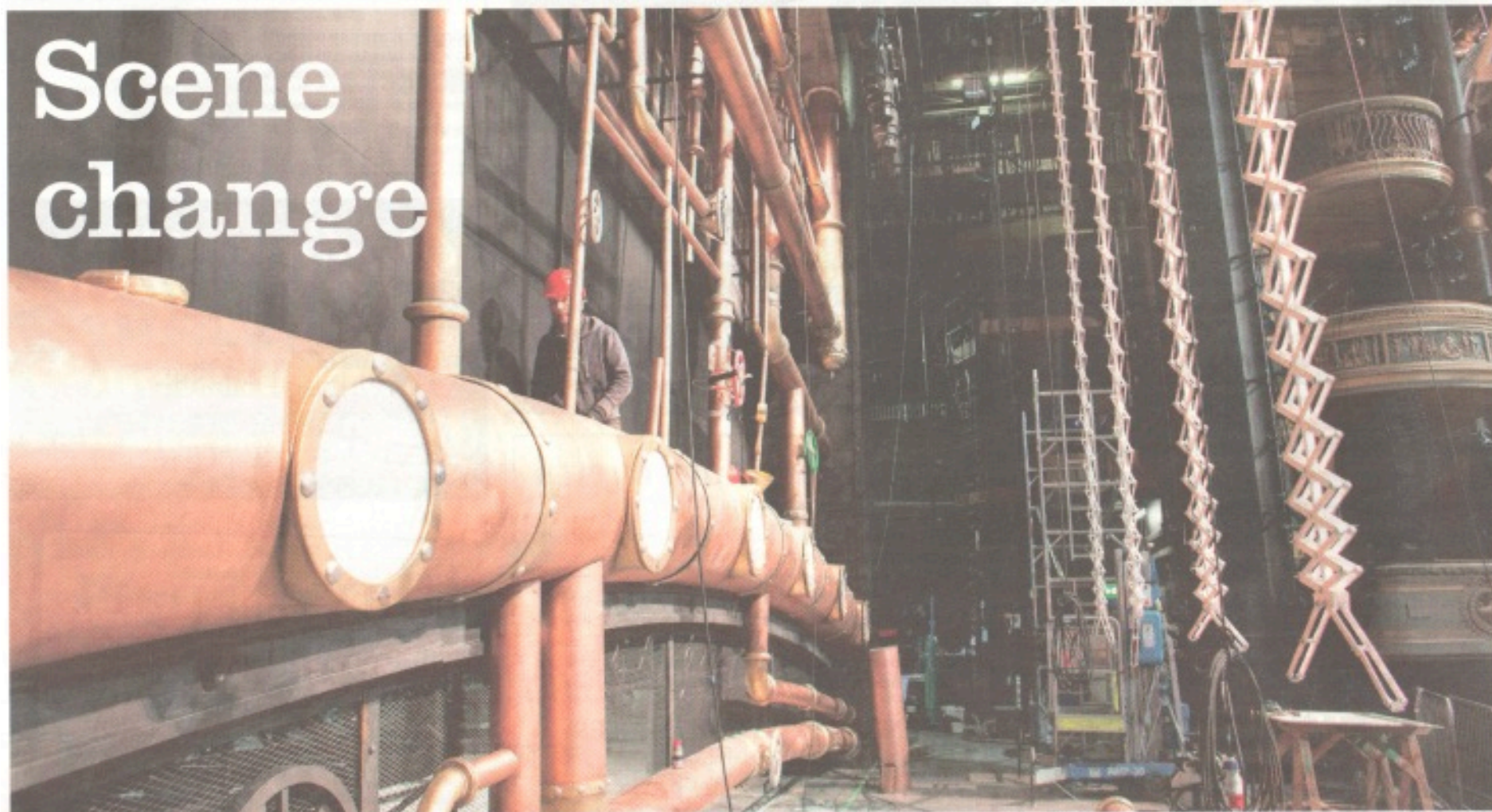
Installing some of the 13 tons of beam trusses used in Charlie and the Chocolate Factory at Theatre Royal Drury Lane, London
